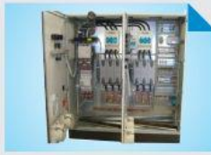
Therister Control Panels
